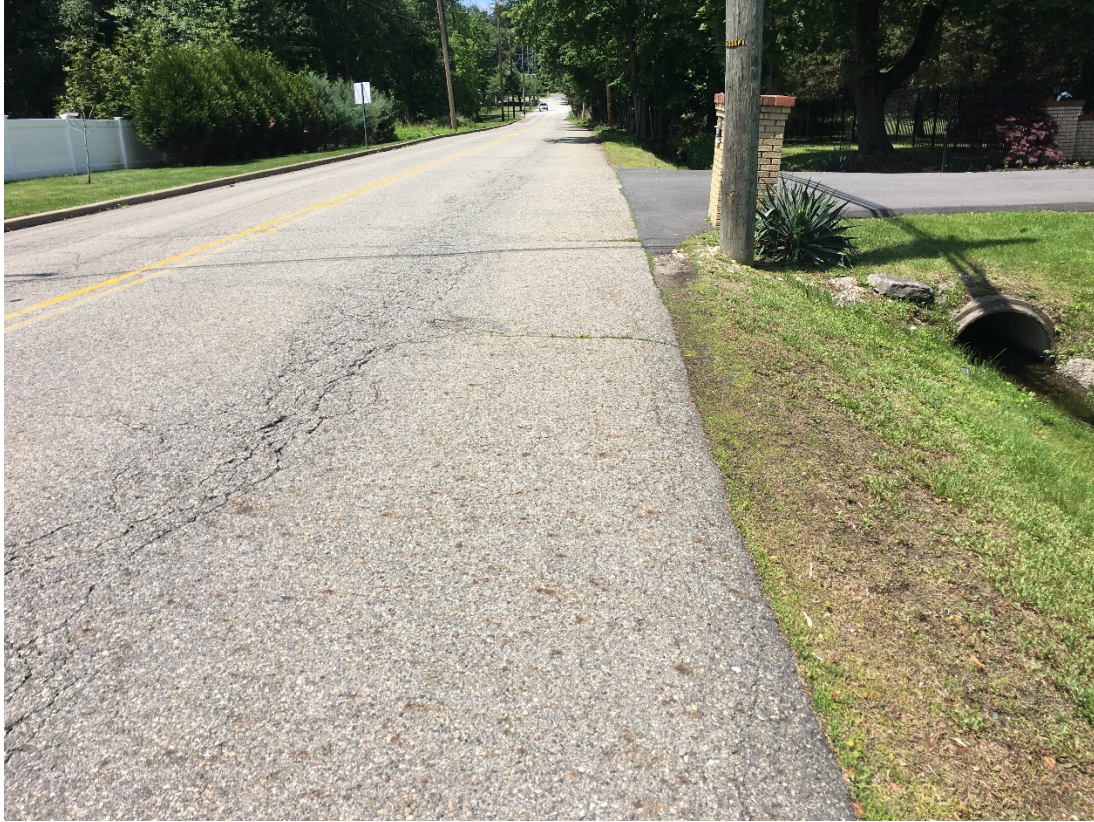
View looking westerly down Sunset Road showing unconfined pavement edge, drainage ditch and rutting in westbound travelled way.
