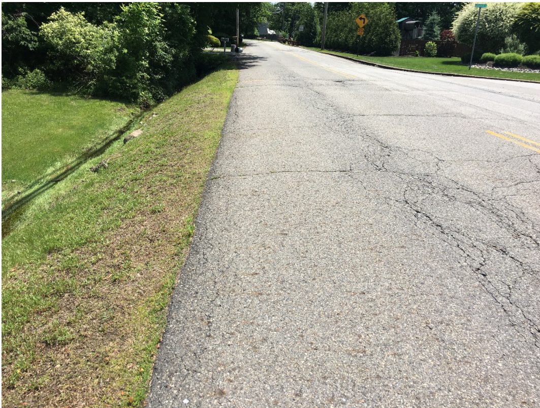
View looking easterly down Sunset Road showing unconfined pavement edge, drainage ditch and rutting in westbound travelled way.
