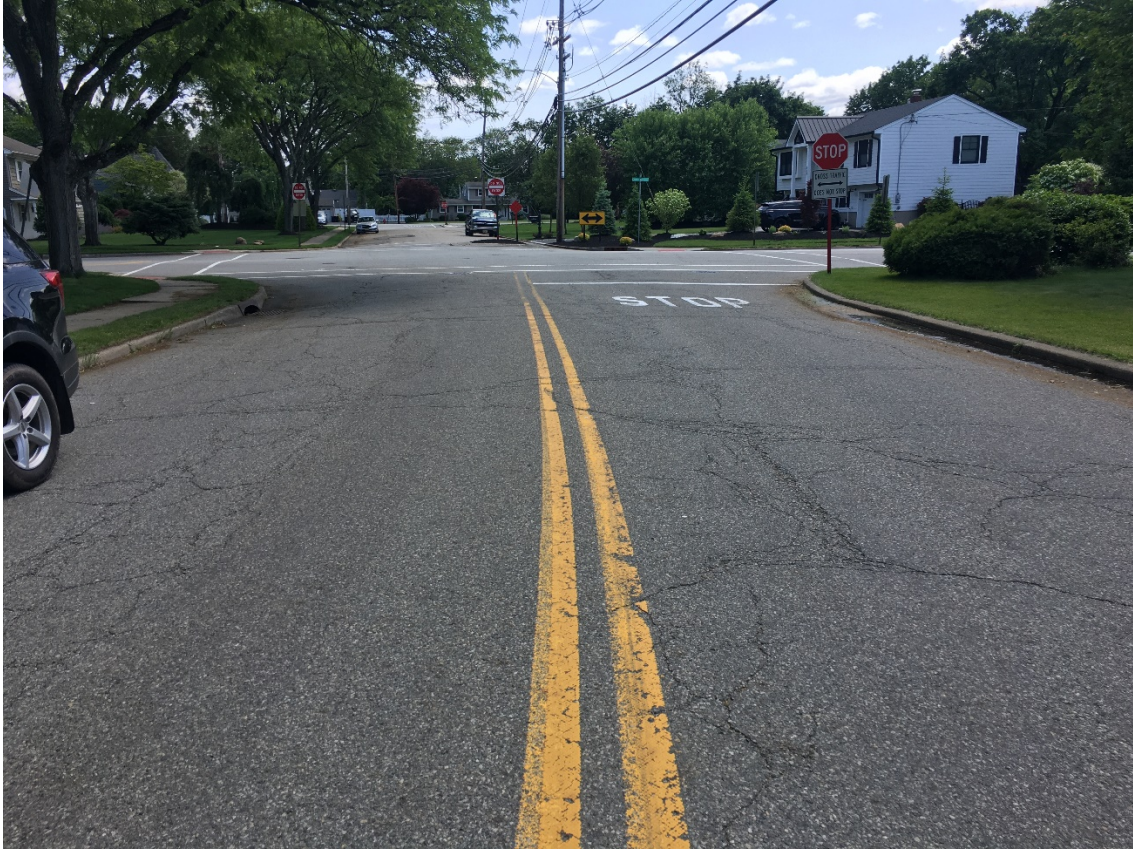
View looking easterly across West Parkway/Sunset Road intersection. Note localized drainage issue along curbline.
