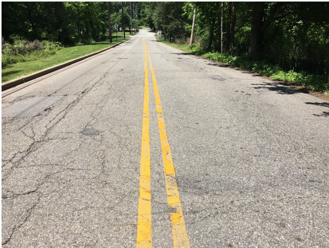
View looking westerly down Sunset Road showing unconfined pavement edge and rutting in travelled way.
