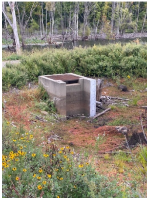
Figure 3a. Overflow Box
